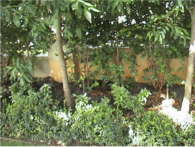
Stained white stucco walls
